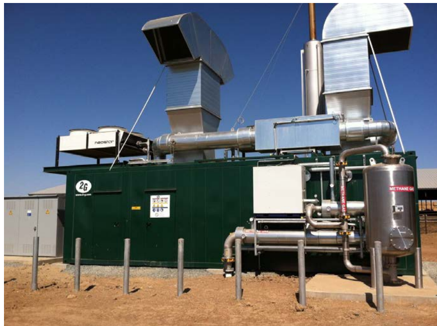
Figure 7: New Hope 450 kW Engine-Generator
